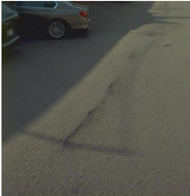
Rutting along with Raveling
