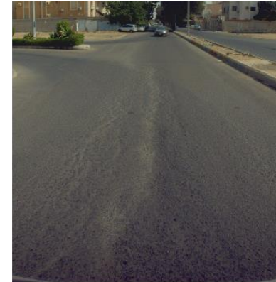
Severe weathering and raveling
