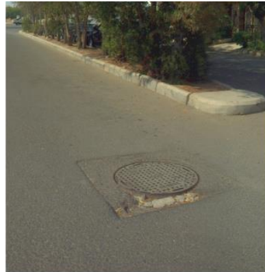
Poor patch around manhole
