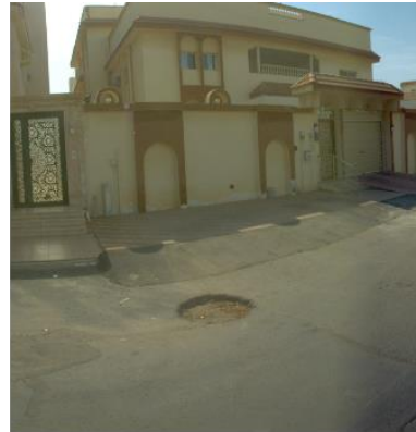
Depression in manhole
